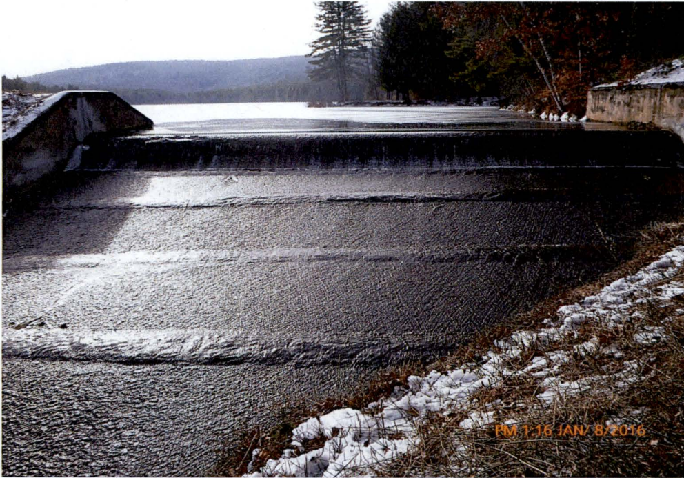
Photo 3 Dam ID# 188-0783 Woodward Lake Dam 01/08/2016 Service spillway's downstream face and upper discharge chute as observed from the spillway's left side. Notice repairs made to cover joints in the discharge chute.
