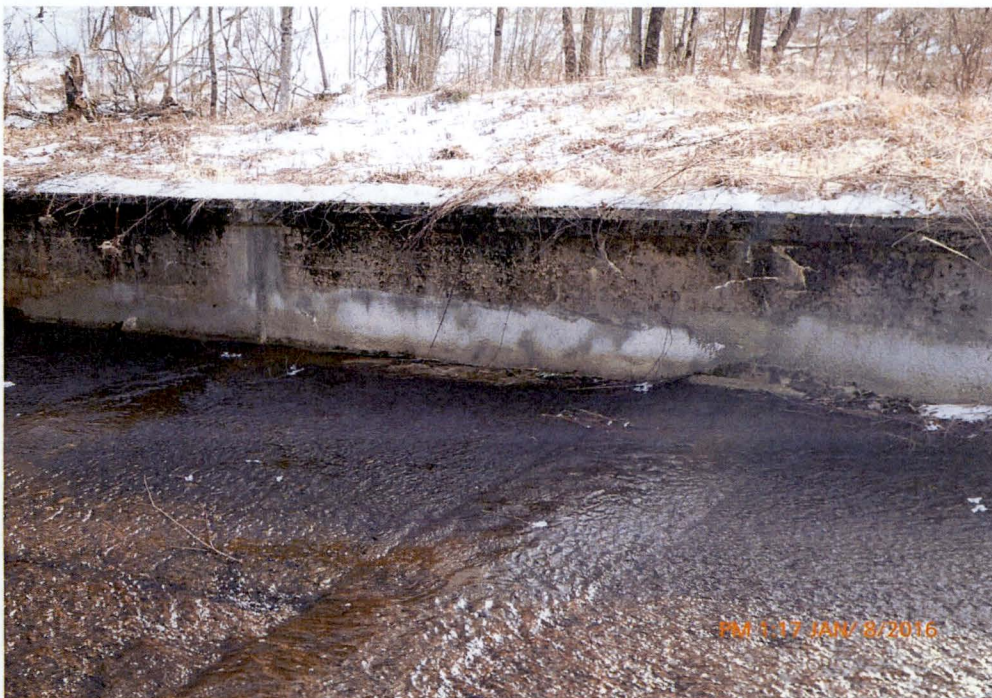
Photo 4 Dam ID# 188-0783 Woodward Lake Dam 01/08/2016 Service spillway's right downstream training wall as observed from the service spillway's left downstream side. Notice concrete repairs made to wall.
