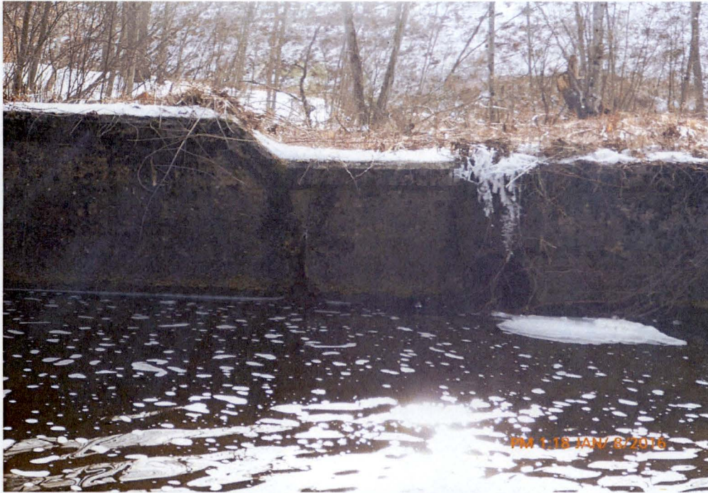
Photo 7 Dam ID# 188-0783 Woodward Lake Dam 01/08/2016 Low level outlet conduit's discharge end and a crack( minor void) in the base of service spillway's right downstream training wall as observed from the service spillway's left downstream side.
