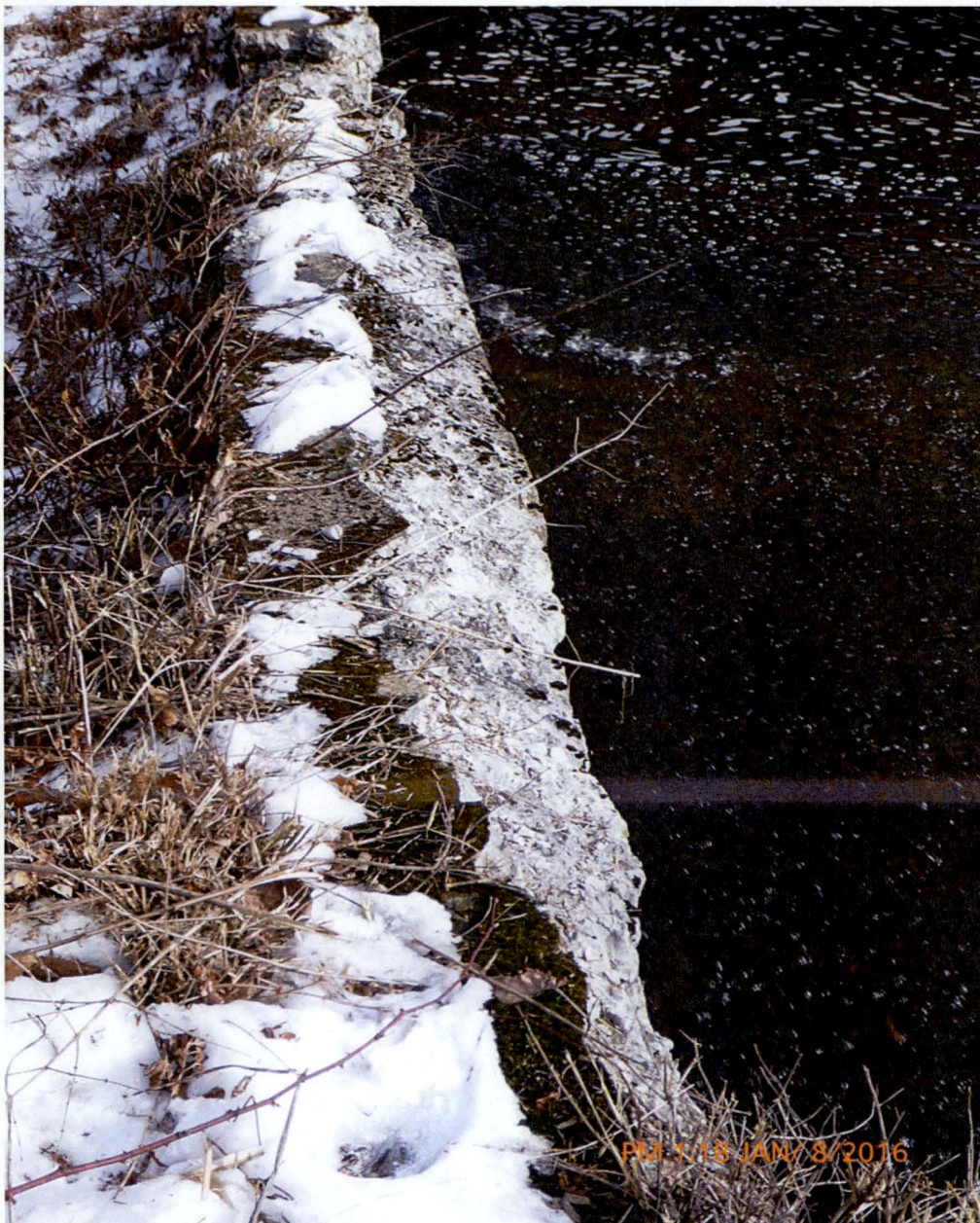
Photo 6 Dam ID# 188-0783 Woodward Lake Dam 01/08/2016 Concrete deterioration of the left service spillway's downstream training wall as observed from the service spillway's left side
