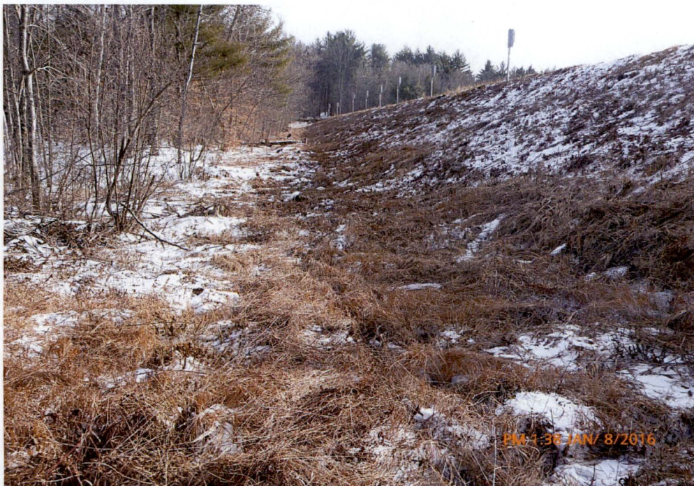
Photo 16 Dam ID# 188-0783 Woodward Lake Dam 01/08/2016 Right embankment's downstream toe as observed from the service spillway's right side.
