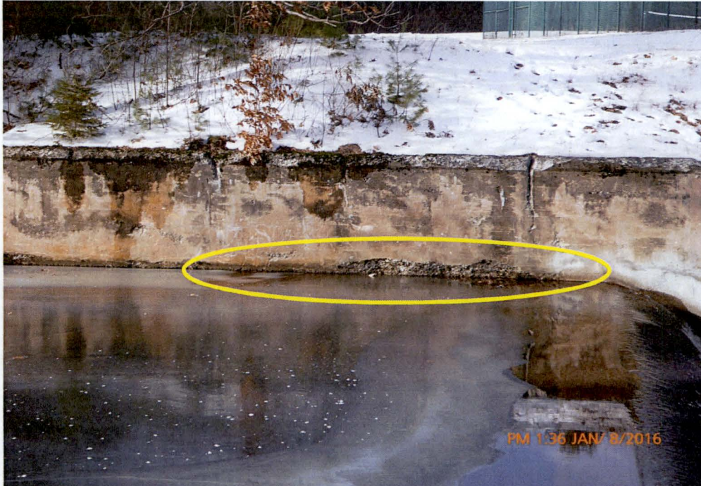
Photo 14 Dam ID# 188-0783 Woodward Lake Dam 01/08/2016 Concrete deterioration at the water line - service spillway's left upstream training wall as observed from the service spillway's right side.
