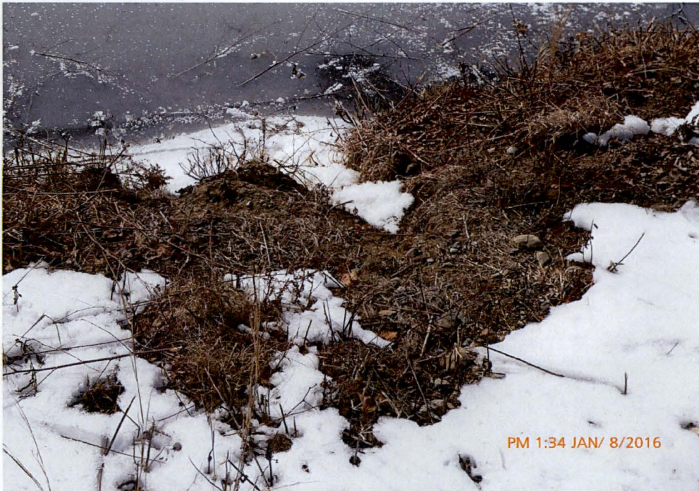
Photo 12 Dam ID# 188-0783 Woodward Lake Dam 01/08/2016 Wave erosion observed on the right upstream embankment as observed from the embankment's crest.
