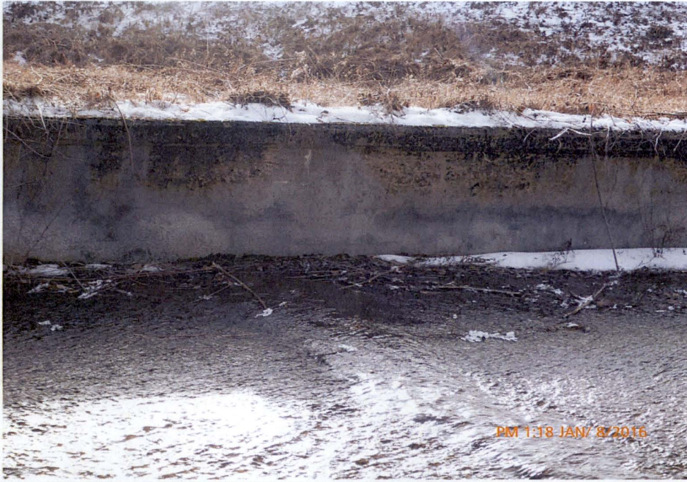
Photo 5 Dam ID# 188-0783 Woodward Lake Dam 01/08/2016 Minor concrete deterioration at base of service spillway's right downstream training wall as observed from the service spillway's left downstream side. Also observe concrete maintenance performed on the training wall.
