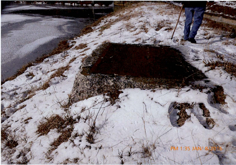
Photo 13 Dam ID# 188-0783 Woodward Lake Dam 01/08/2016 Concrete vault observed on the dam's right embankment. Vault was locked but believe to house the low level outlet valve.
