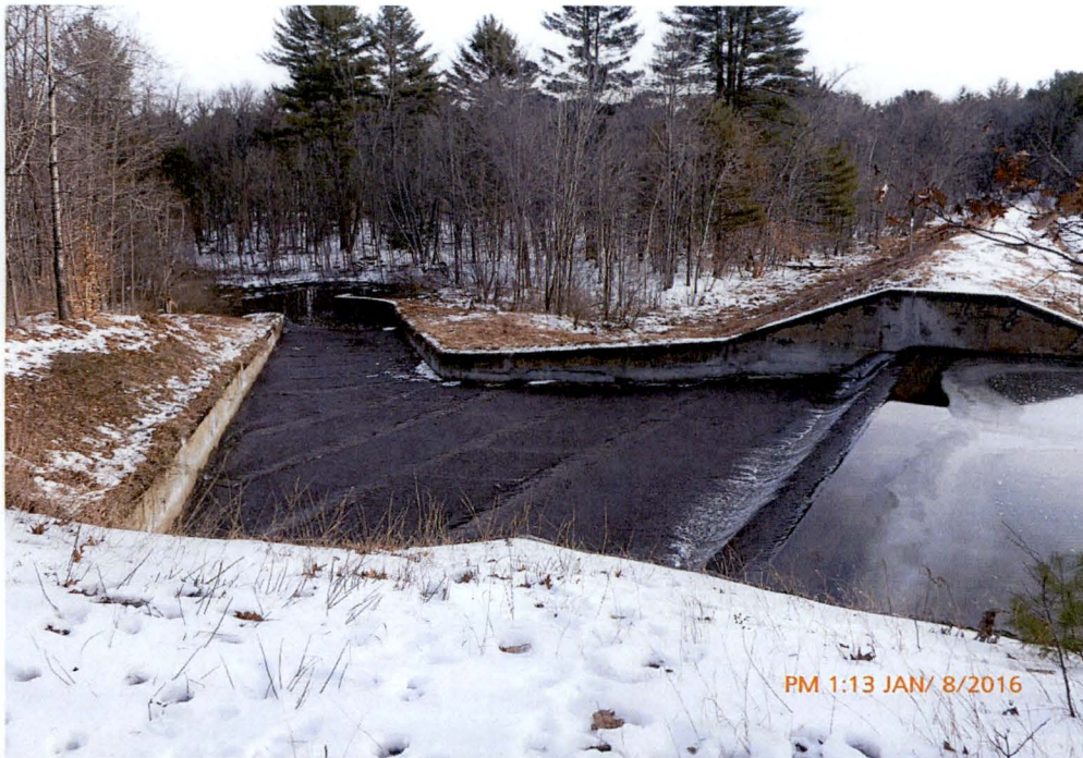
Photo 1 Dam ID# 188-0783 Woodward Lake Dam 01/08/2016 Service spillway, service spillway's right training wall, spillway discharge chute, and right embankment section as observed from the spillway's left side.
