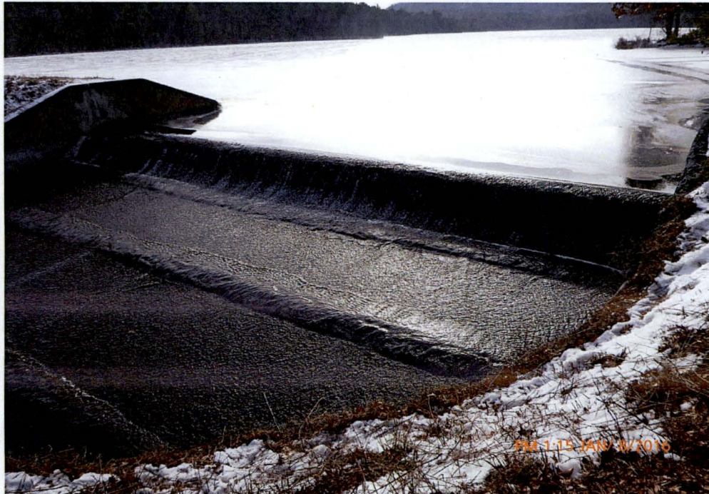
Photo 2 Dam ID# 188-0783 Woodward Lake Dam 01/08/2016 Service spillway's downstream face and upper discharge chute as observed from the spillway's left side. Notice repairs made to cover joints in the discharge chute.
