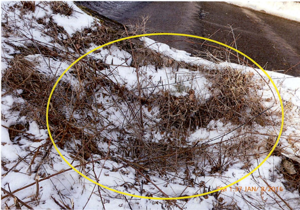
Photo 15 Dam ID# 188-0783 Woodward Lake Dam 01/08/2016 Depression observed adjacent to service spillway's right downstream training wall. The depression was located at the embankment's downstream toe
