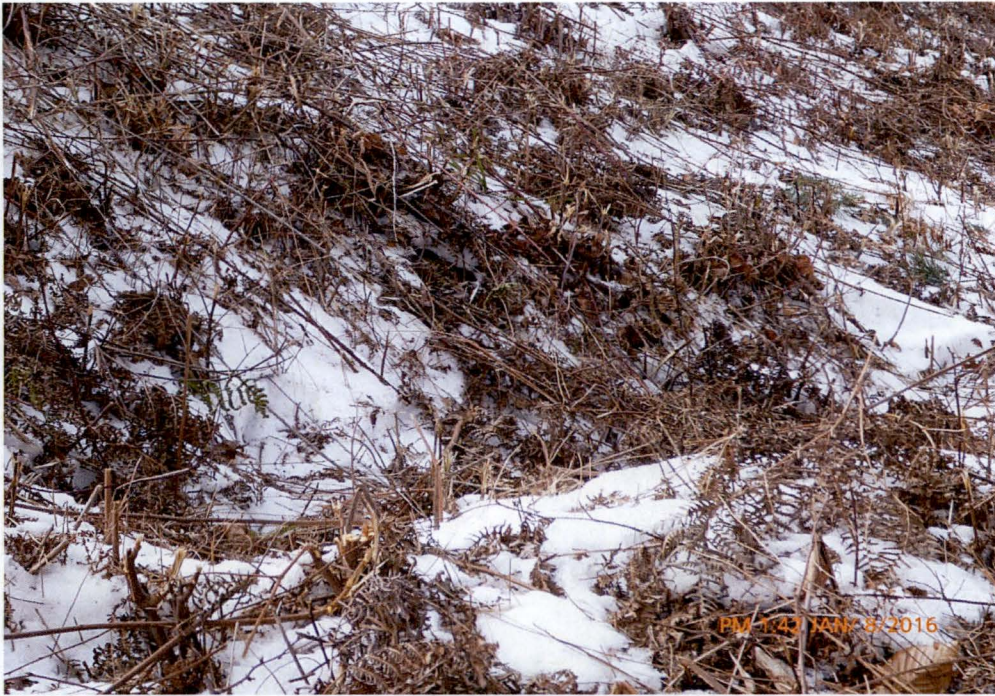
Photo 19 Dam ID# 188-0783 Woodward Lake Dam 01/08/2016 Minor depression / slough on the right downstream embankment as observed from the embankment's toe.
